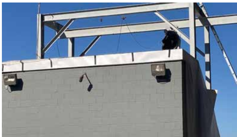
The newly painted and refurbished pump building and hoist system is shown above. Work also included a new roof on the building.
