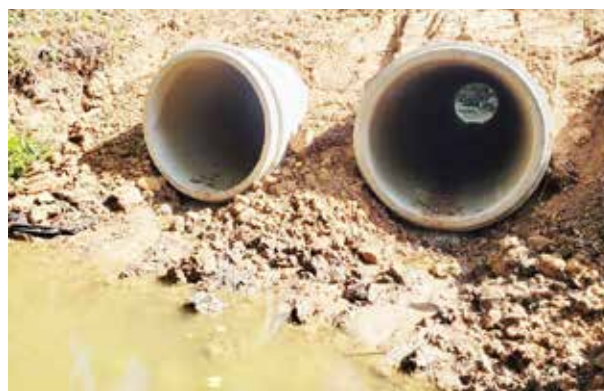
GRAVITY DRAINAGE CANALS UPGRADED... A $400,000 project to add 60 inch concrete culverts in the Gravity Drainage District is complete. The project was completed with grant funds and will re-establish drainage in the Atchafalaya Basin, which will benefit the Morganza floodway.
