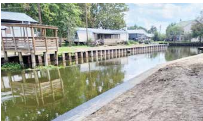
DISCHARGE BAYOU BULKHEAD REPAIRS... A contractor recently completed bulkhead repair of the outflow channel at Discharge Bayou and Lighthouse Canal under direction of the parish. The bulkheads had begun to fail and were at the end of their life expectancy.
