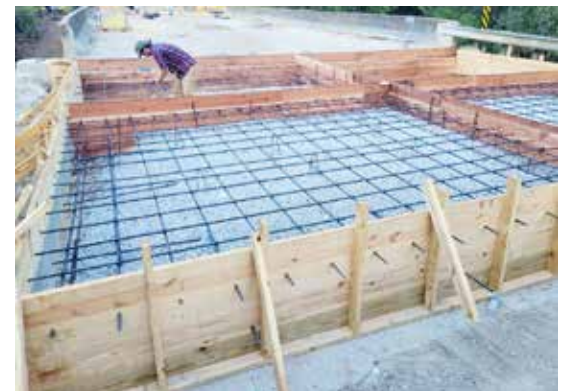
JACK TORRES BRIDGE REPAIR UNDERWAY... The embankment of the bridge is being rebuilt. One third of the road was overlaid two years ago, and the remainder of the road will be overlaid in 2025.
